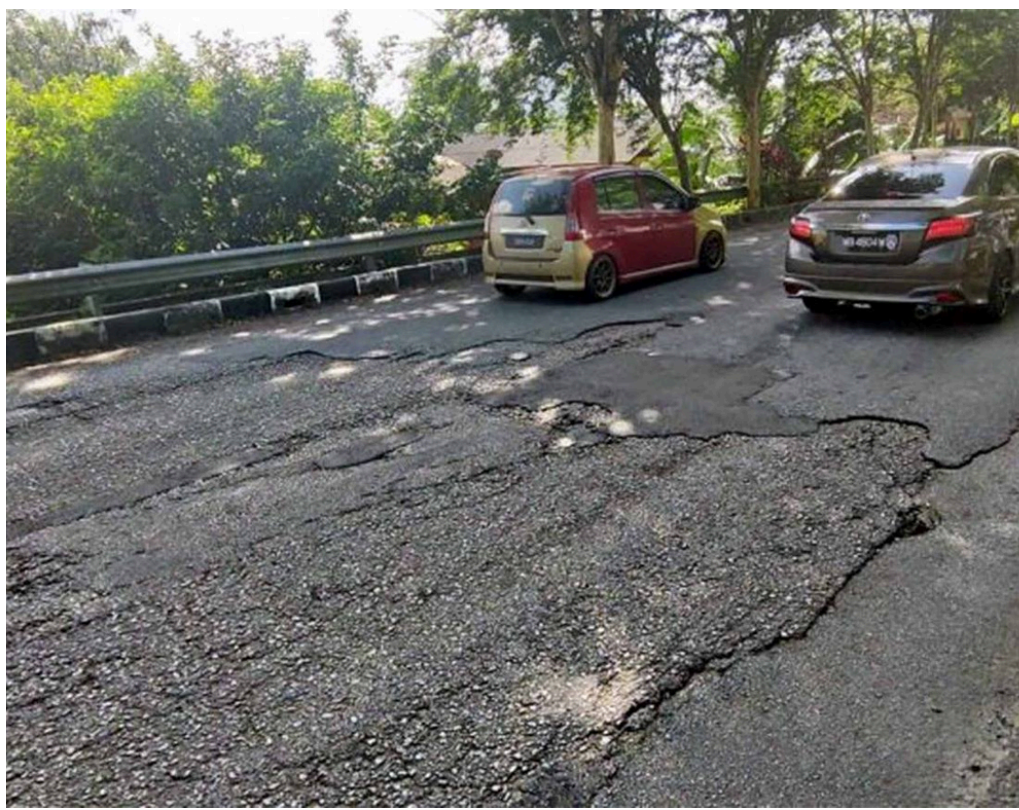
POOR ROAD CONDITIONS
